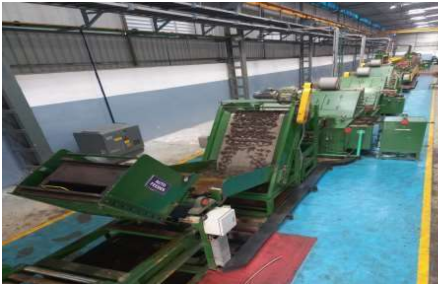
Heat Treatment Section Equipped with 3 PLC Controlled Continuous Mesh Belt Furnaces
