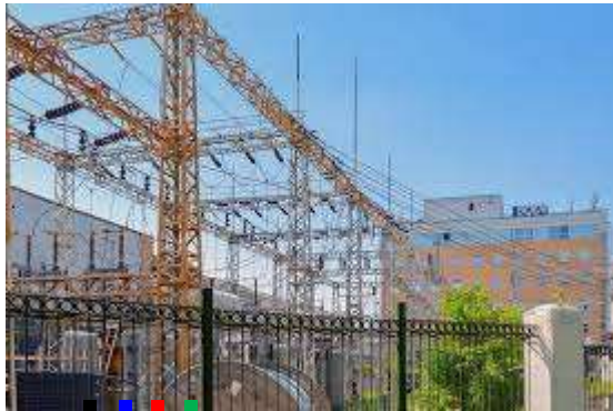
Factory main power line
